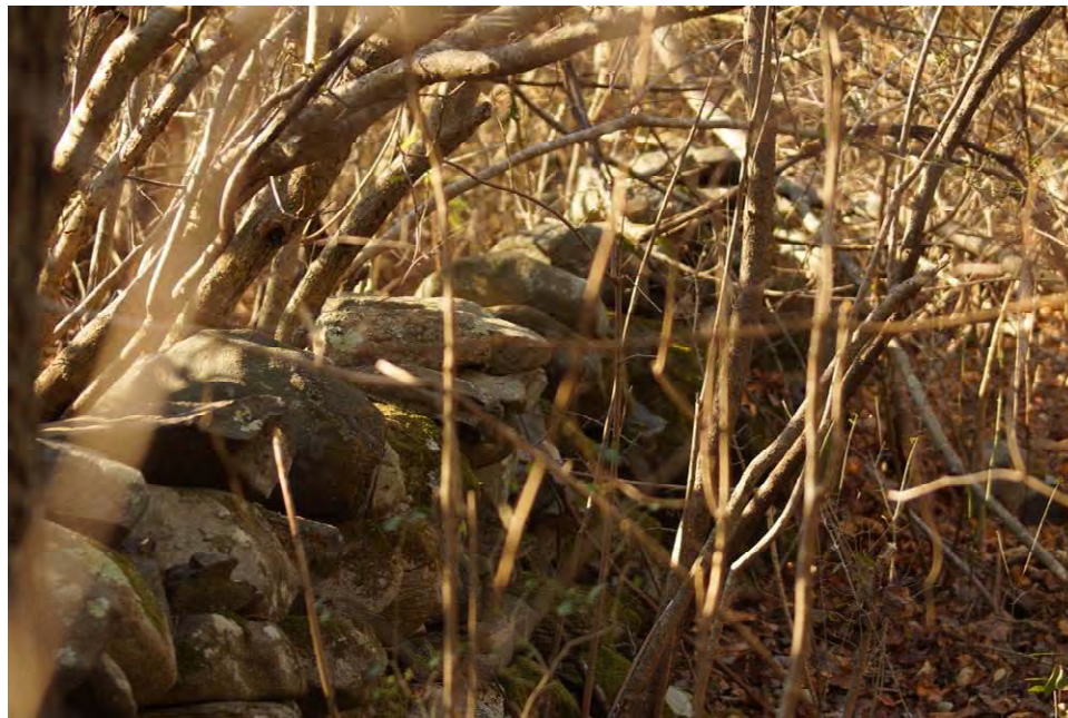
Figure 8. Representative photographs of stone walls, Canonchet Farm Bike Path Extension Feasibility Study Area.
